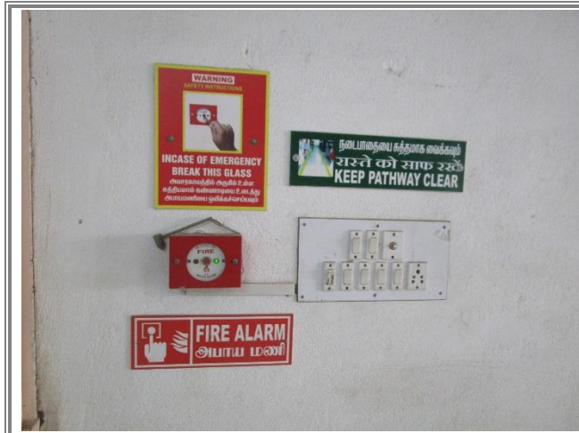
Fire alarm call point
