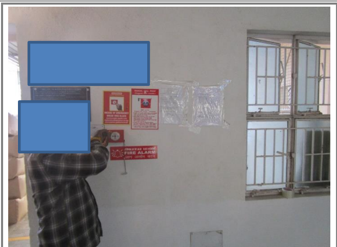
Fire alarm tested
