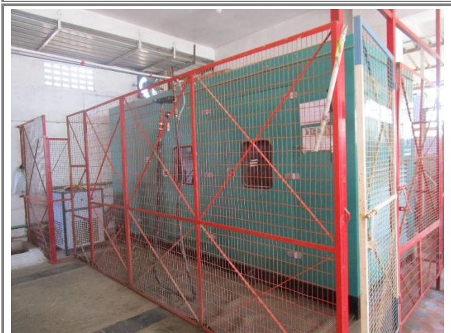
Diesel generator area
