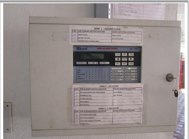
Fire alarm control panel
